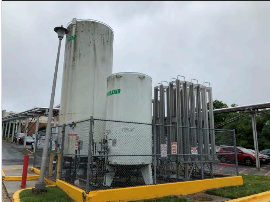
17 - Hospital oxygen storage
