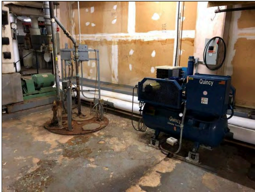
8 - Air compressor, sump pump
