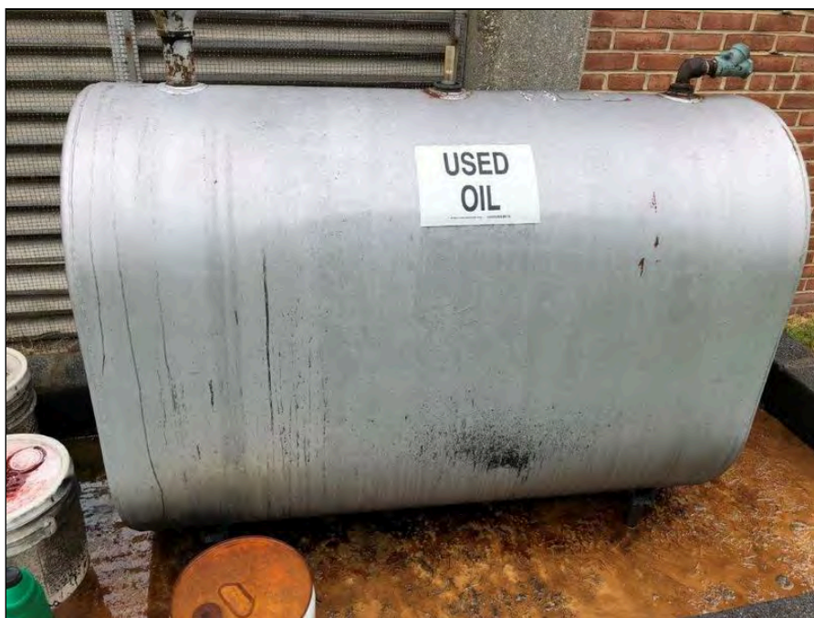
22 - 275-gallon used oil AST
