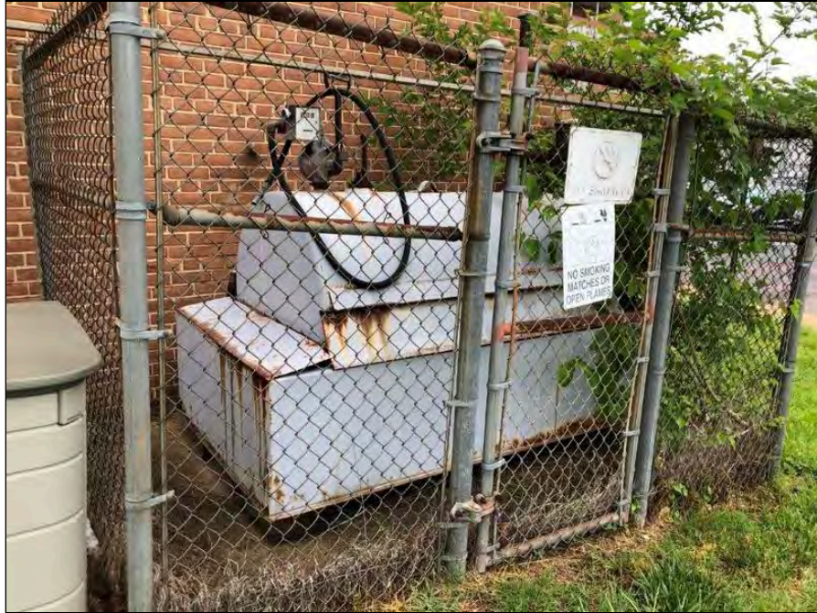
25 - Suspect 500-gallon fuel oil AST
