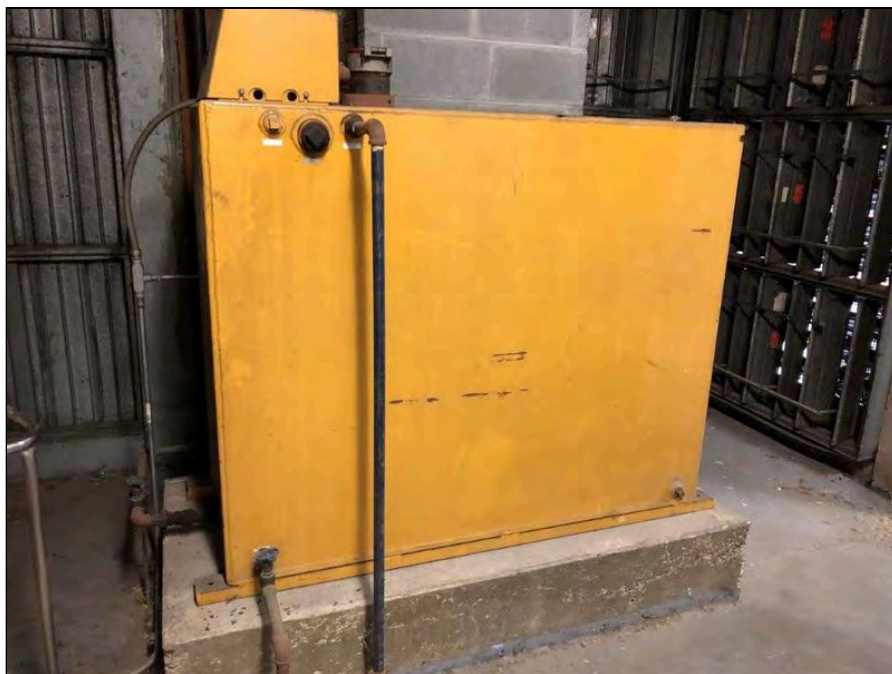
11 - Emergency generator diesel fuel storage
