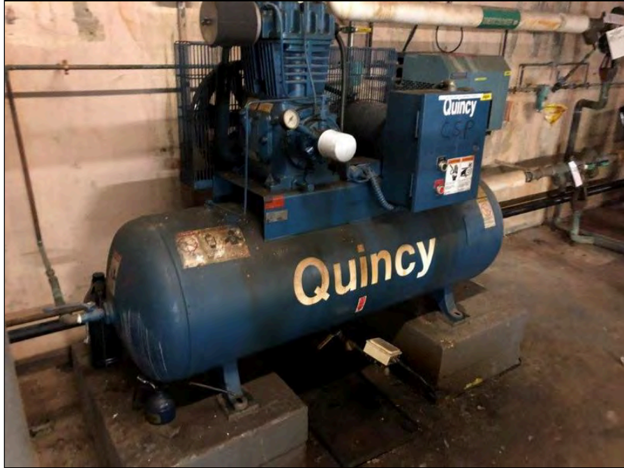
7 - Representative air compressor, staining
