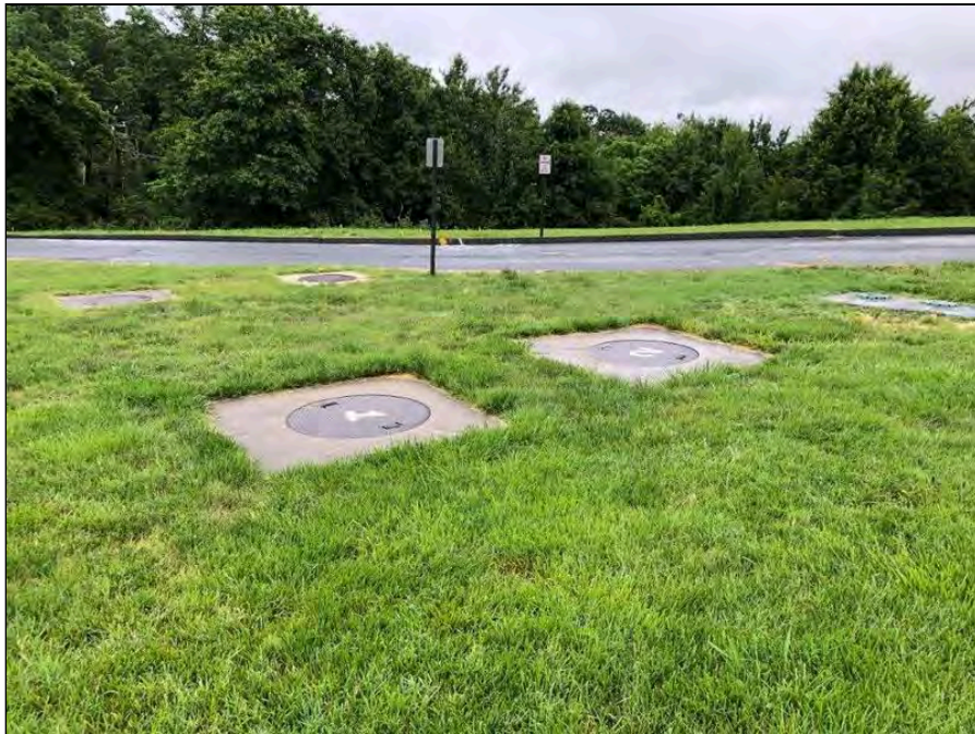
24 - Two 20,000-gallon heating oil USTs
