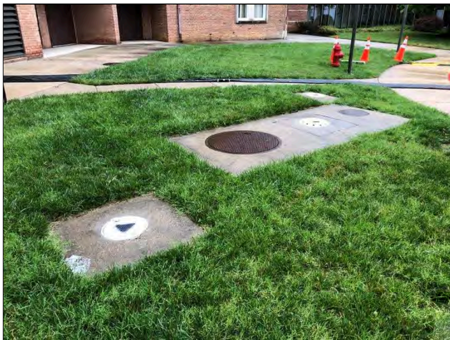
19 - Suspect 5,000-gallon diesel fuel UST
