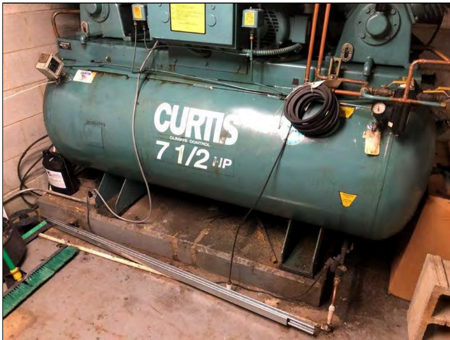
6 - Representative air compressor
