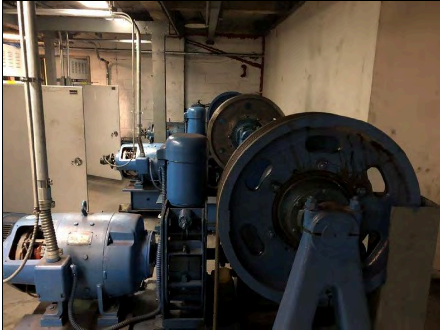
5 - Traction wheel elevator room
