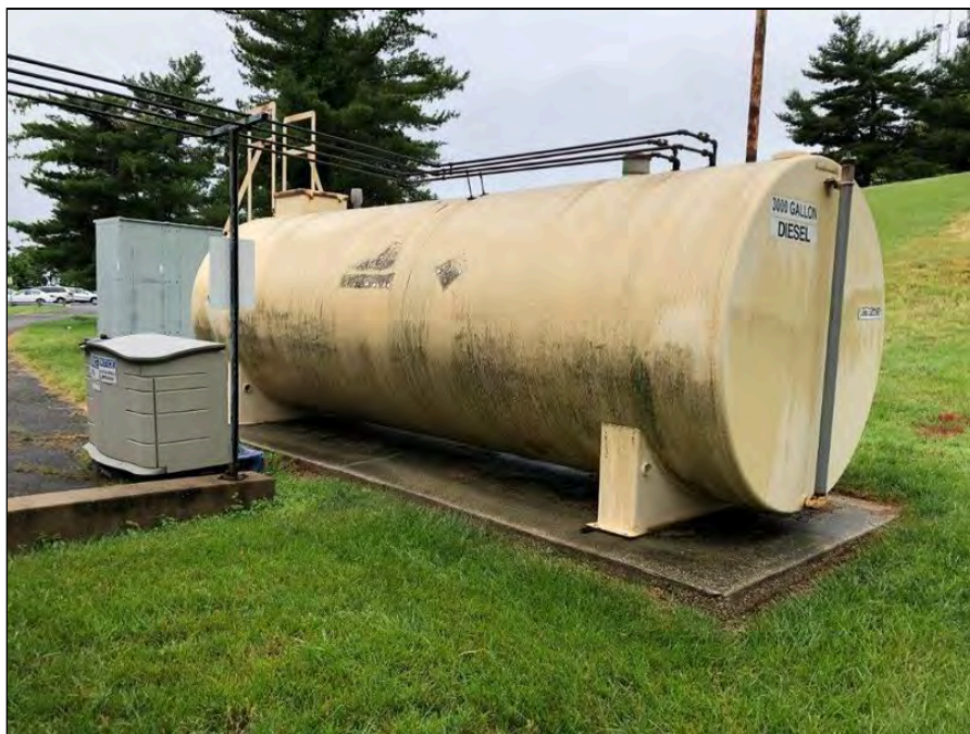
20 - 3,000-gallon diesel fuel AST
