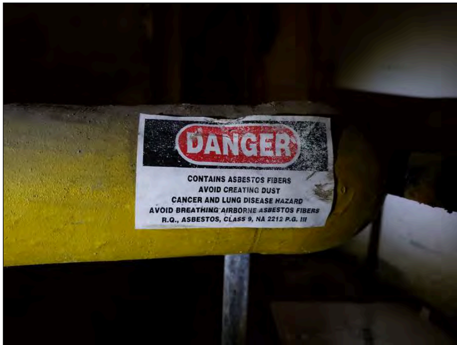
8 - Asbestos Labels Observed
