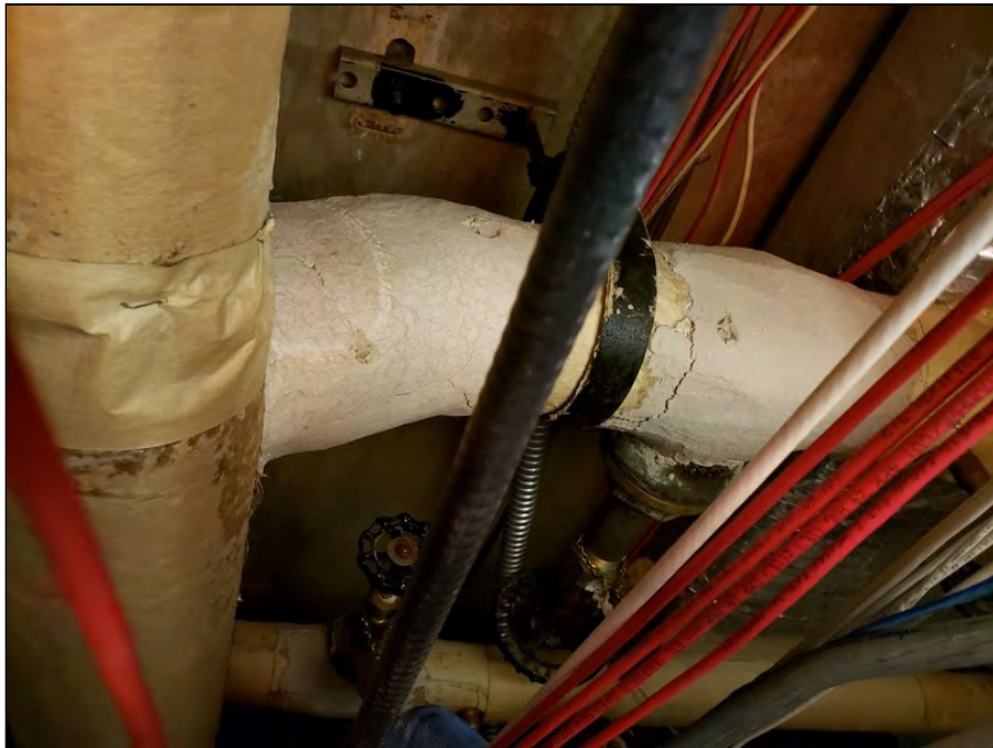
2 - Cemented Pipe Elbow (ACM)
