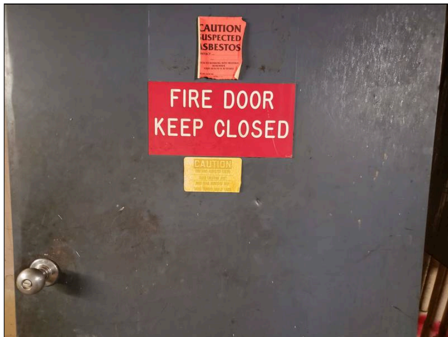
5 - Fire Door and Frame (Suspect ACM)
