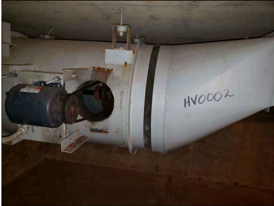
9 - Vibration Dampener (Suspect ACM)
