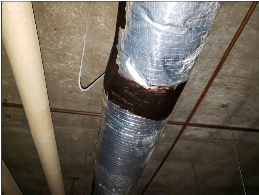
4 - Black Duct Mastic (ACM)
