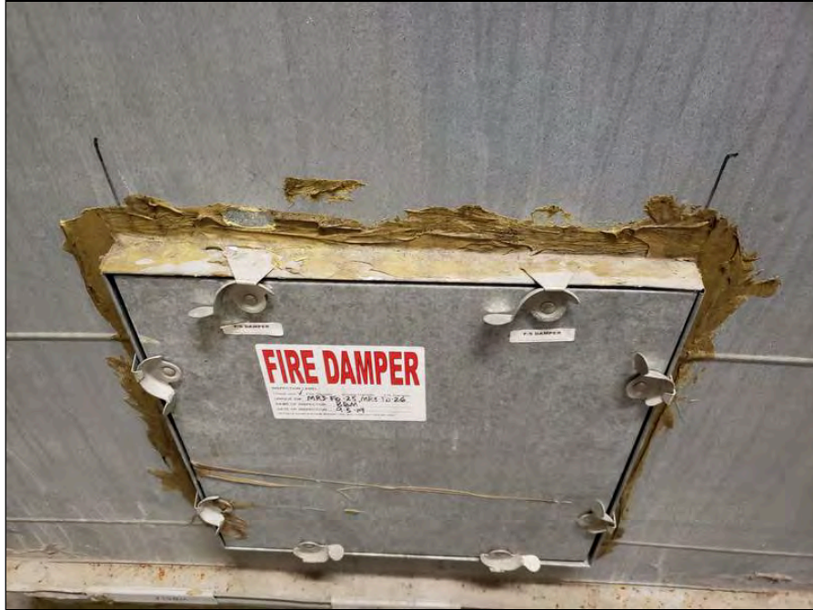
7 - Fire Damper (Suspect ACM)
