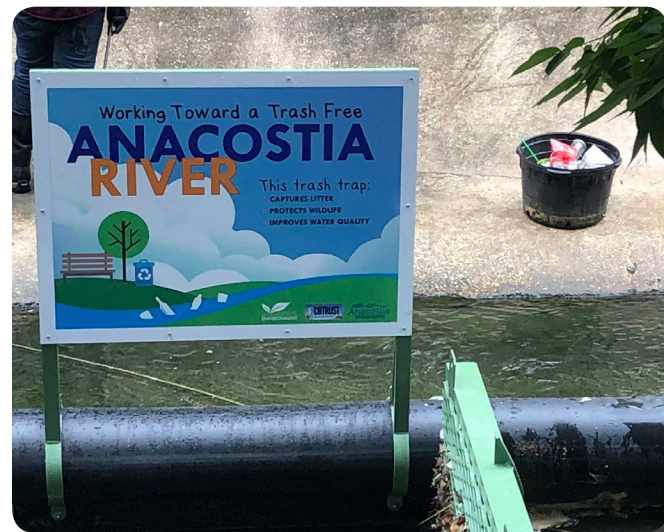
Installation of a Bandalong Litter Trap in Mount Rainier, MD in 2018 was funded by a Stormwater Stewardship Grant and made possible by many community partnerships.
