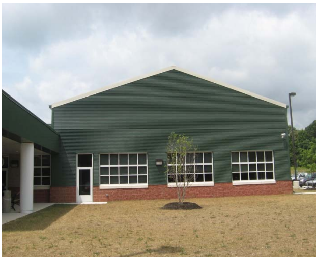
Exterior view from the east of the Canine Holding Kennel Area – exterior finishes are durable and appear to have held up well over the seven years since the building opening
