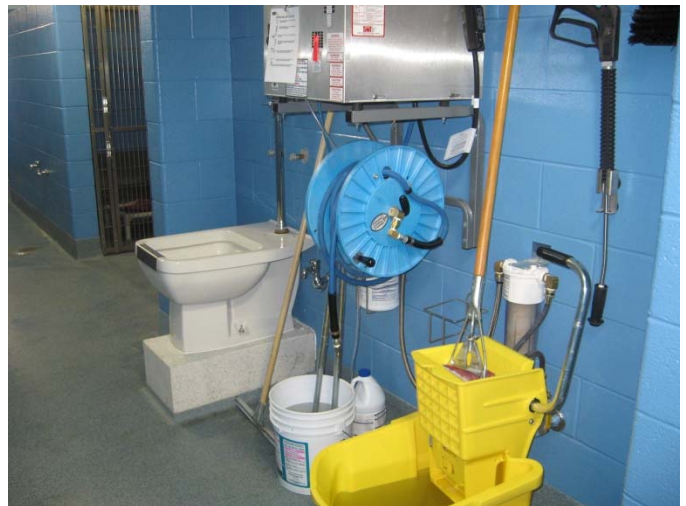
Clinic sink and high-pressure wash-down system (note, this photo was taken when the facility originally opened, materials no longer look as new – see photo above for comparison)
