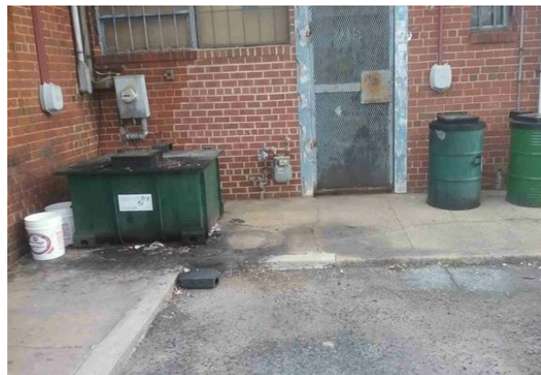
Grease container spillage
