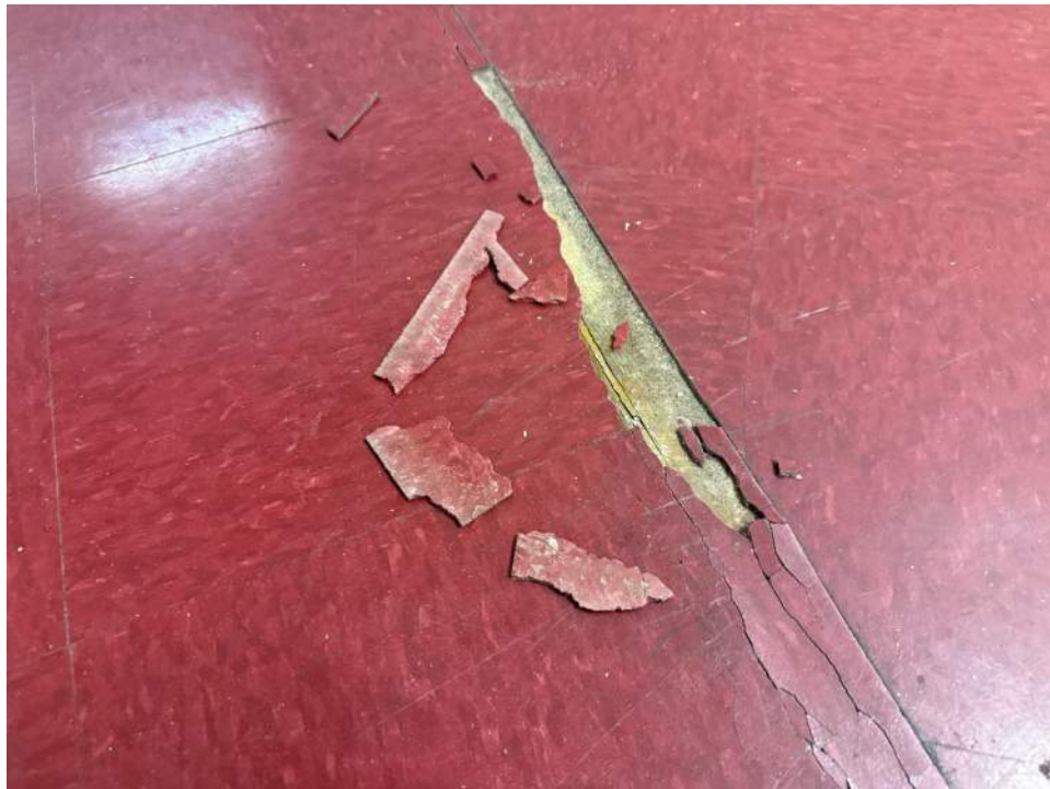
Photo 8 – Failure in Level 3 floor finish
