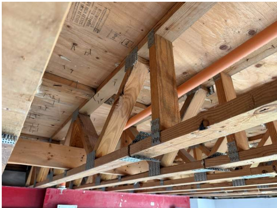
Photo 4 – Wood connection bottom splice plate failures
