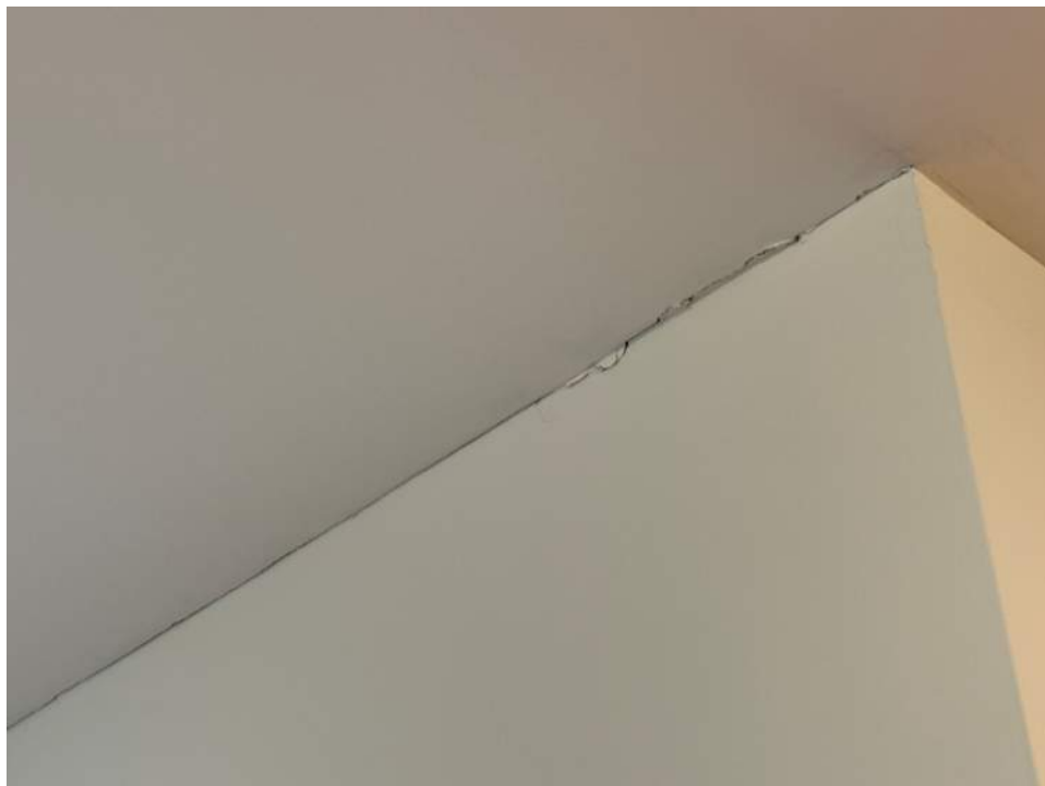
Photo 10 – Crack at Unit 305 wall/ceiling transition
