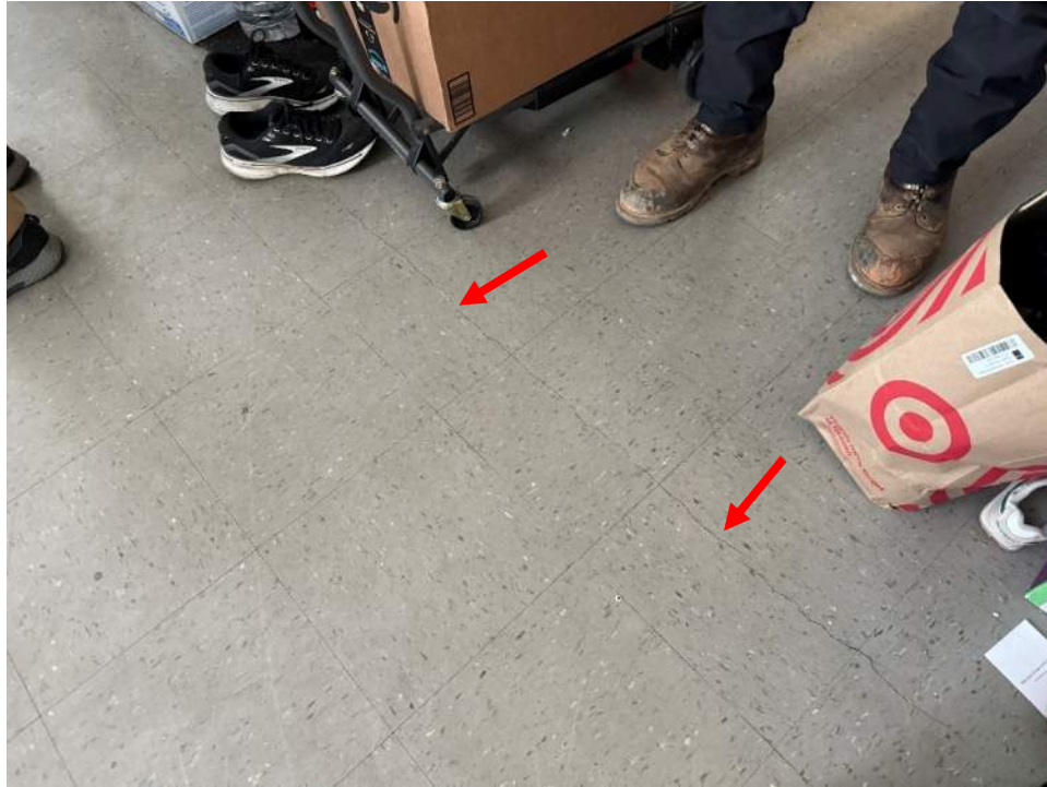
Photo 7 – Unit 312 floor finish cracks
