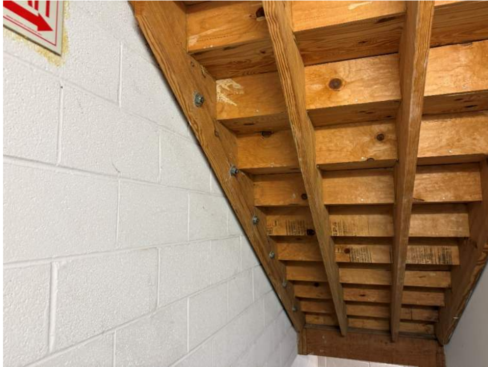
Photo 11 – Stair stringer with skewed anchors
