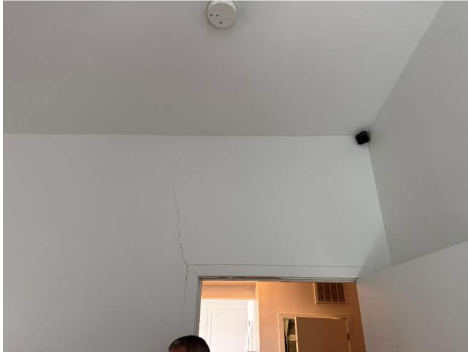
Photo 9 – Crack propagating from Unit 305 door header/jamb corner
