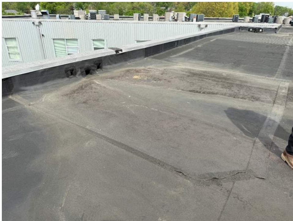
Photo 14 – Overview of roofing area with failed patch repairs
