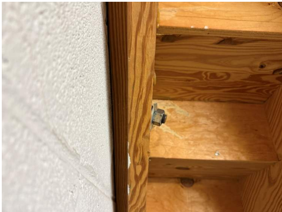
Photo 12 – Stair stringer with skewed anchors
