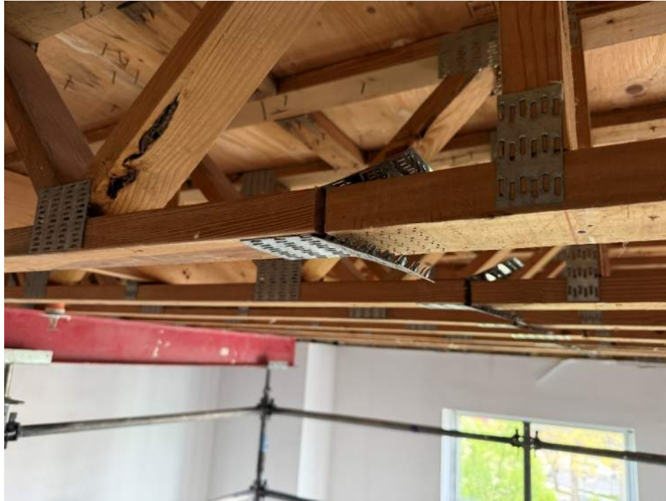
Photo 5 – Wood connection bottom splice plate failures
