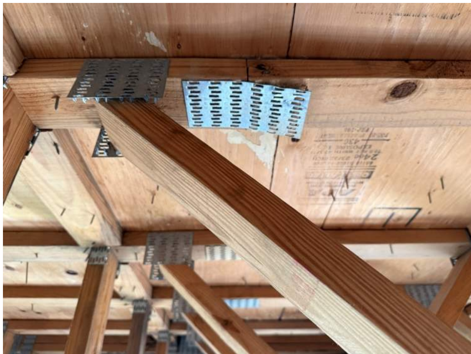
Photo 6 – Top splice and adjacent diagonal connection plate failures
