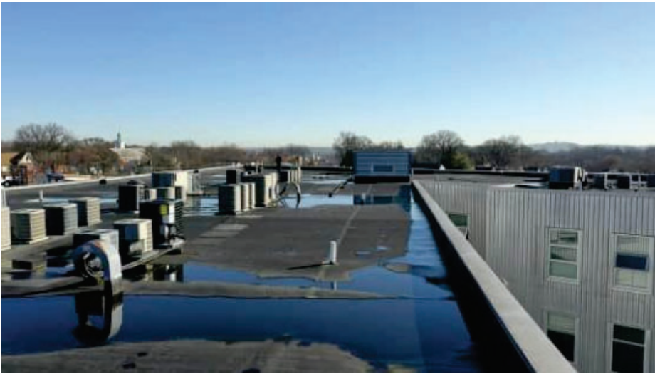
Major ponding on entire roof
