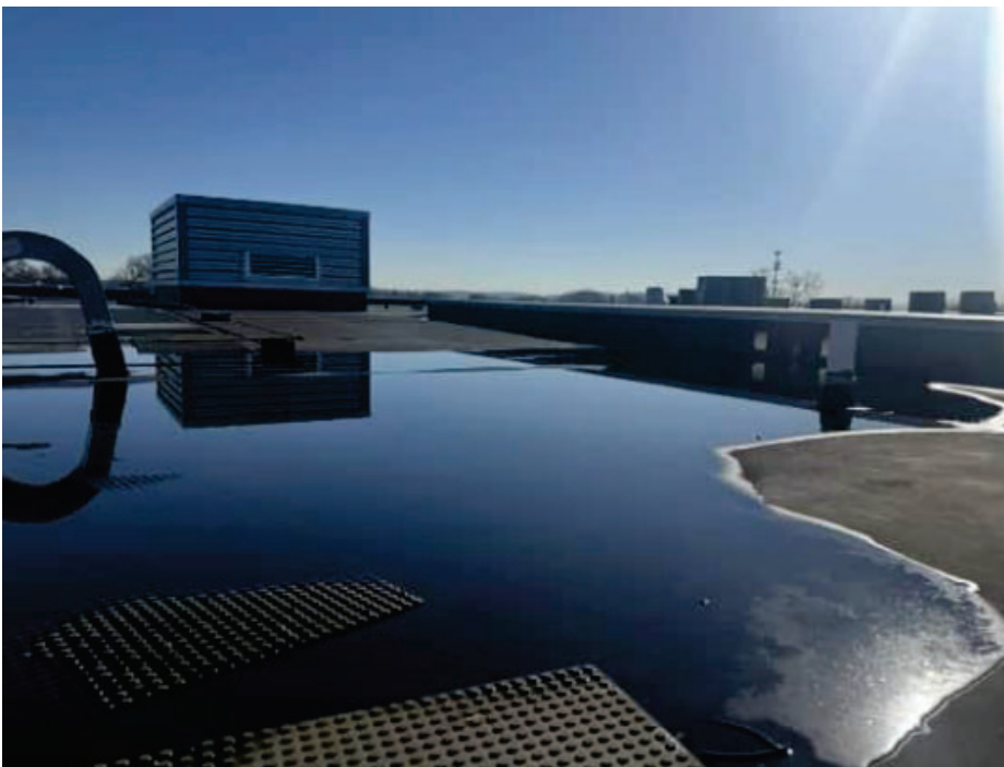
Inadequate slope for proper drainage
