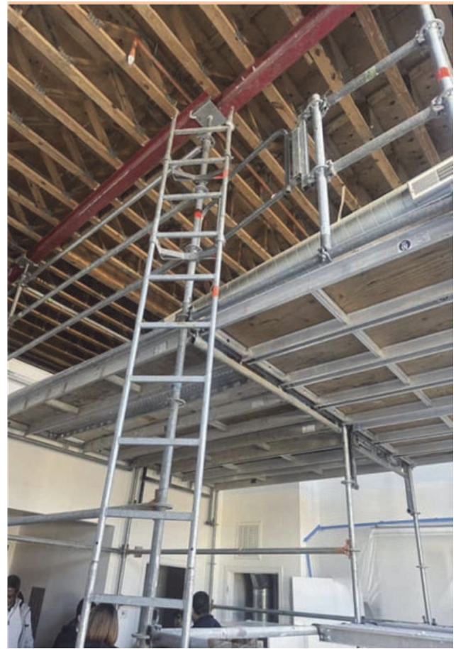
Picture showing temporary support of failed ceiling trusses
