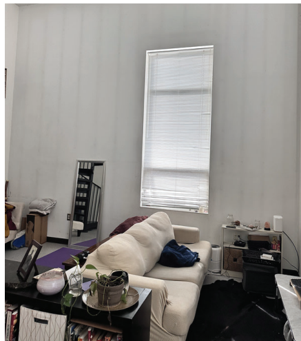
Ghosting repainting required
