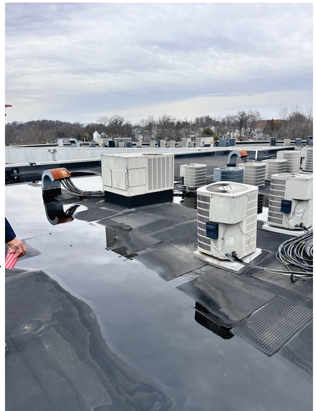
Picture showing rooftop units with exposed wires
