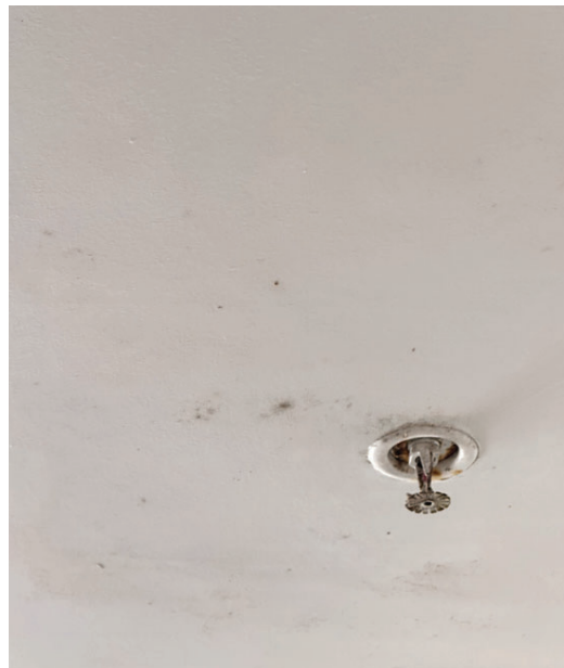
Defective and non-functional sprinkler systems
