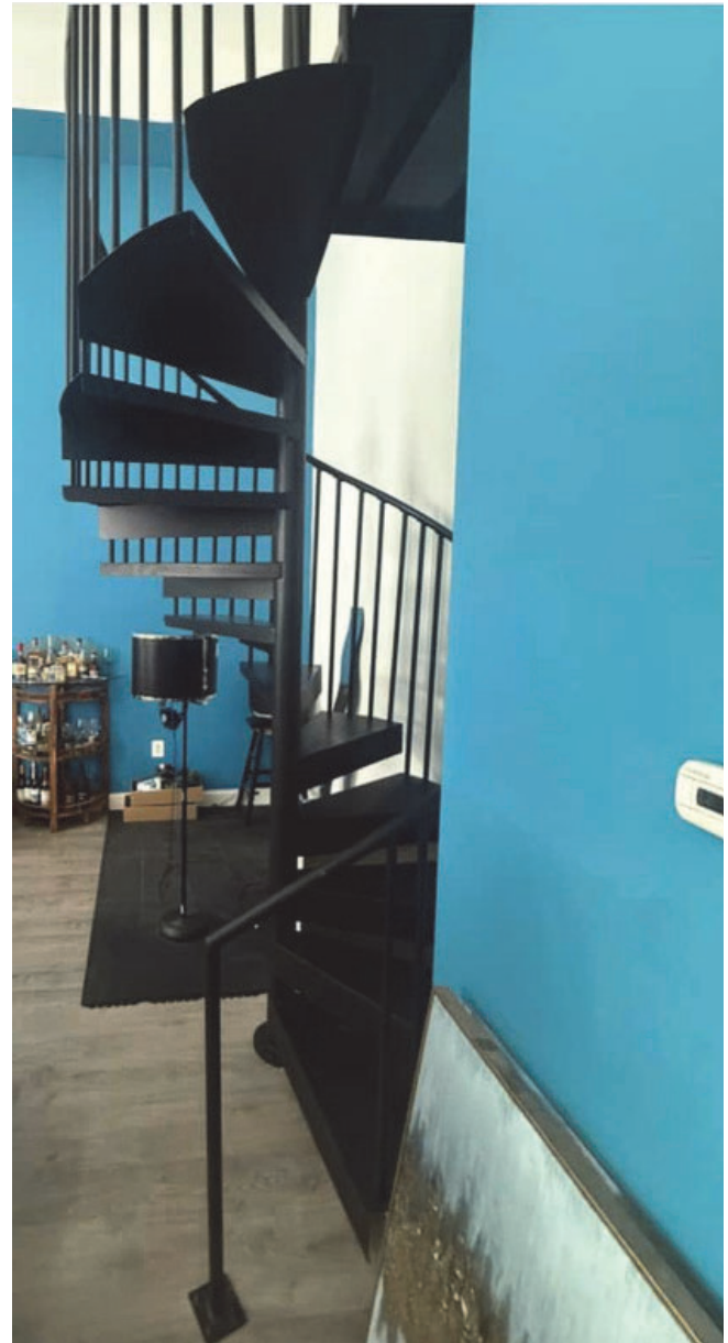
Illegal spiral staircase installed
