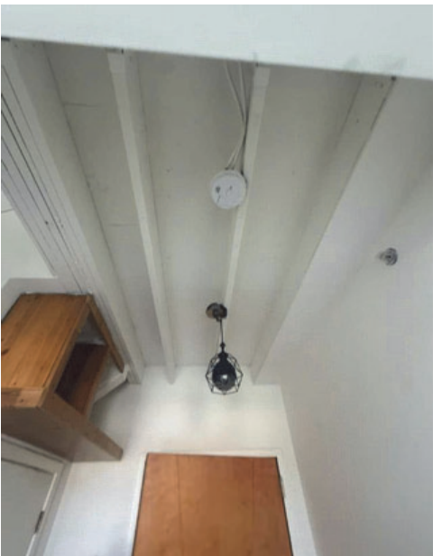
Defective smoke detectors throughout building
