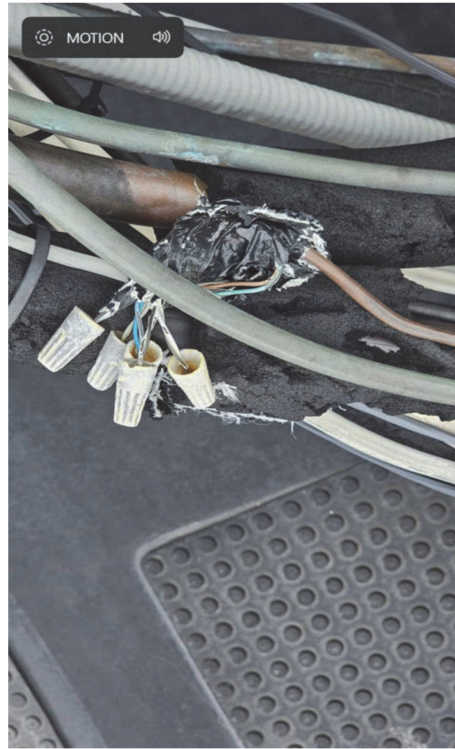
Exposed electrical outlets and lines
