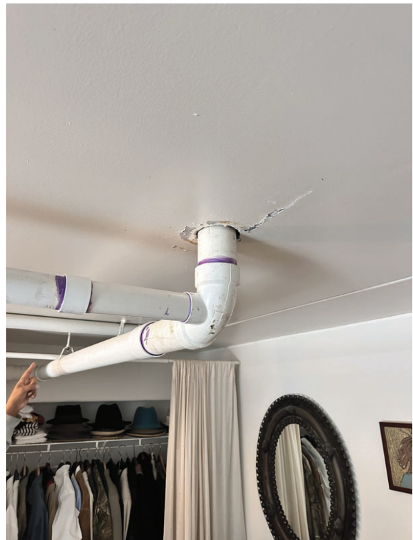
Leaks in residential units
