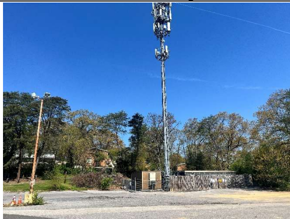
Fenced in telecommunications site
