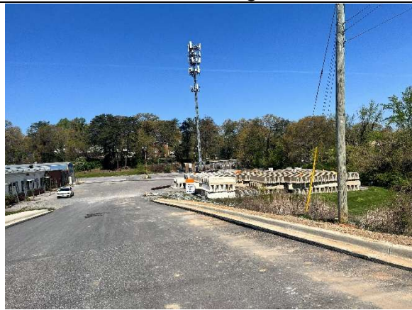
Entrance onto subject property with construction supplies and communications tower at rear of site
