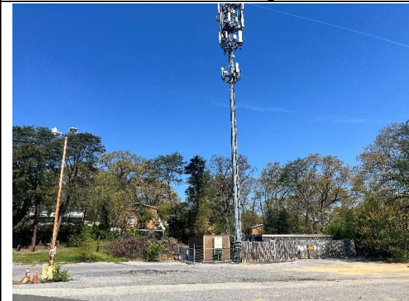
Fenced in telecommunications site
