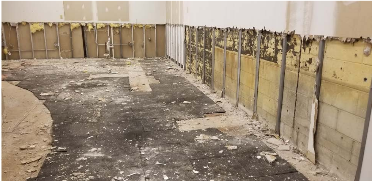
Figure 5.2. Asbestos-containing black wall mastic from a distance.
