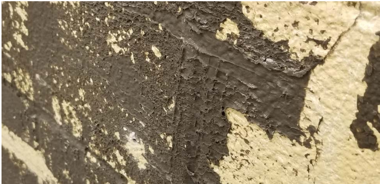
Figure 5.1. Asbestos-containing black wall mastic, close-up.
