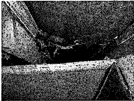
Here you can see the air gap between the insulation and the drywall. Have insulation blown in to fill this gap completely.
