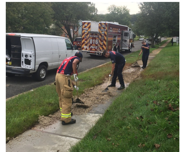
County HAZMAT team puts down absorbents to clean up heating oil.
