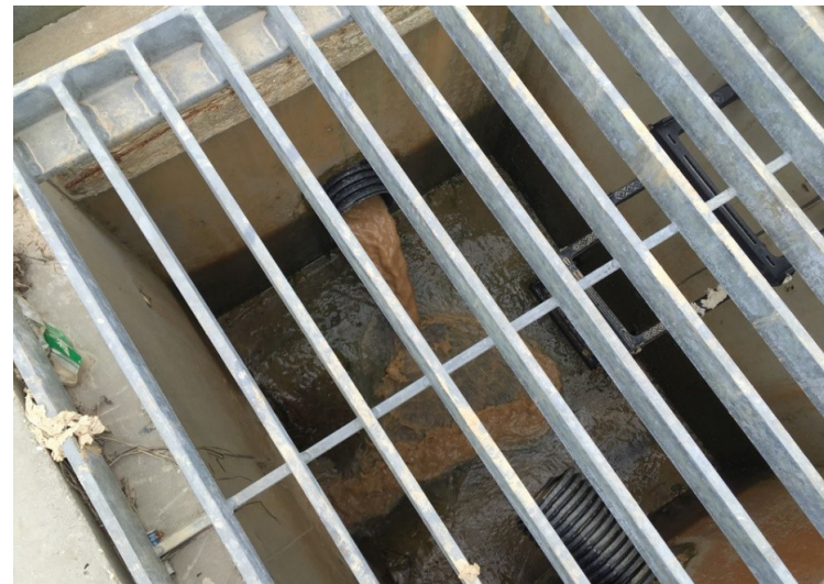
Sediment laden stormwater being discharged into an inlet.
