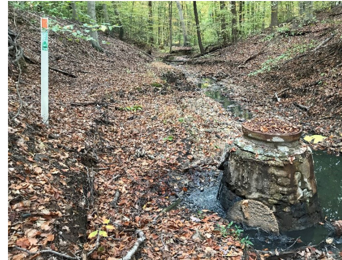
Sewage overflow found in stream. Sewer was unclogged by WSSC.
