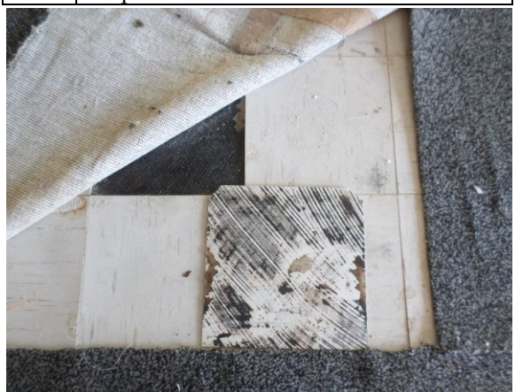
Photo #12: 4622 12x12 White Tile and Mastic #7 and #8 Tile and Mastic ACM
