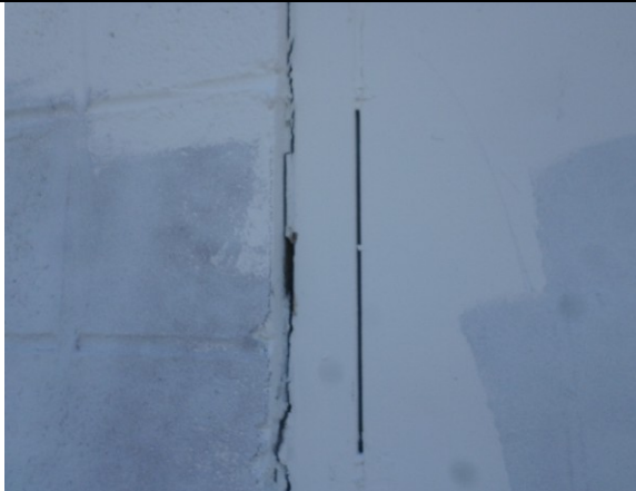
Photo #23: 4626 Rear Door Caulk Sample Set #28 Non-ACM
