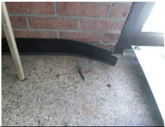
Photo #20: 4626 Main Area 4" Brown Cove Base and Glue Sample Sets #22, #23 Non-ACM
