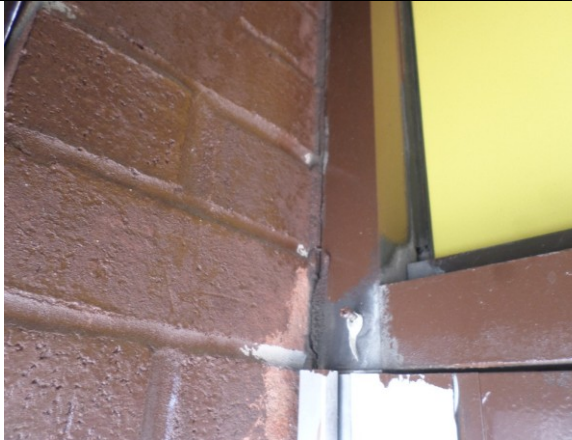
Photo #21: Exterior Window Caulk Sample Set #26 3% Chrysotile
