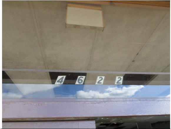
Photo #2: 2x4 Fiberglass ceiling tile
