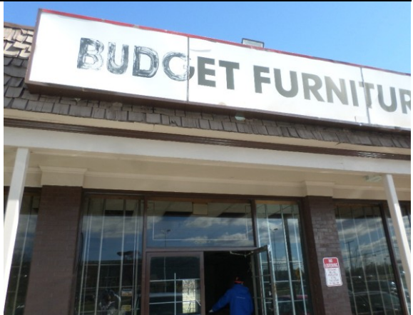
Photo #24: Exterior Window Caulk Sample Set #29 4% Chrysotile
