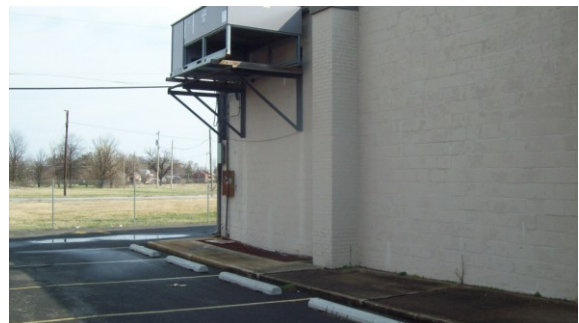
Photo #12: 4646 Exterior Wall Textured Paint Sample 19A Trace <1% Chrysotile Asbestos
