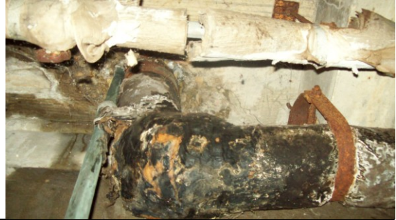
Photo #14: 4646 Basement – Samples 23, 24, 25 ACM Pipe Insulation/Elbows and Seam Cement & Black Mastic on Fiberglass Insulation
