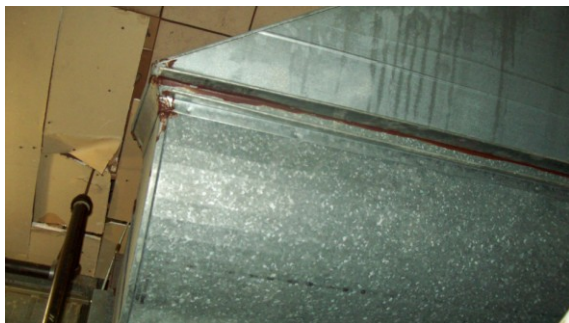
Photo #11: 4646 Hallway-1 Red Duct Seam Sealant Sample 17A Non-ACM
