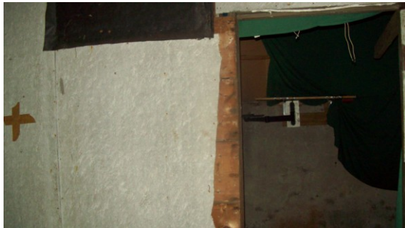
Photo #15: 4646 Basement Cement Wallboard Sample 26A 35% Chrysotile Asbestos
