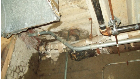
Photo #13: 4646 Basement – Samples 23, 24, 25 ACM Pipe Insulation/Elbows and Seam Cement & Black Mastic on Fiberglass Insulation
