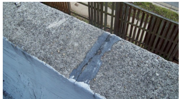
Photo #24: 4670 East Parapet Wall Sealant Sample 41A 5% Chrysotile Asbestos
