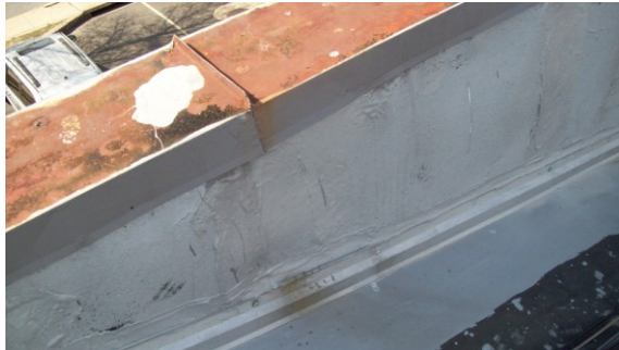
Photo #19: 4646 Roof Flashing Mastic Sample 34A 3% Chrysotile Asbestos
