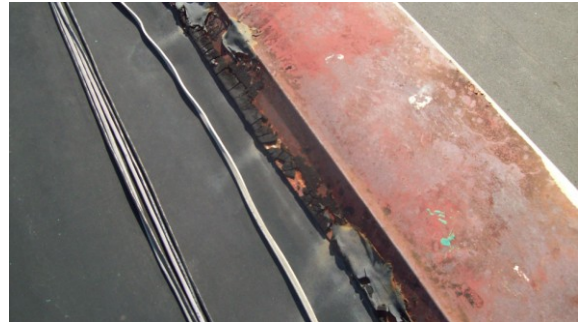
Photo #20: 4646 Roof Tar on Metal Flashing Grey is #5 Chrysotile Asbestos
