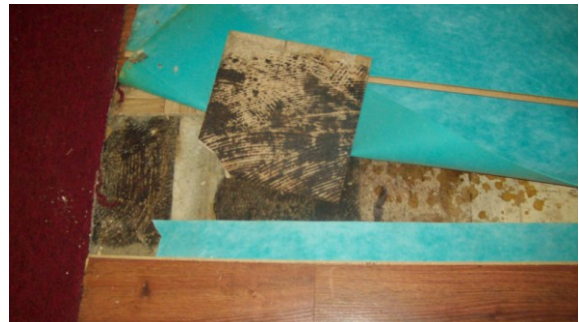
Photo #6: 4646 Under Wood Floor 9'x9' Floor Tile & Mastic Sample Set 8 Tile & Mastic ACM
