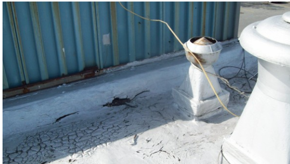
Photo #21: 4670 Roof Flashing and Penetration Tar are ACM
