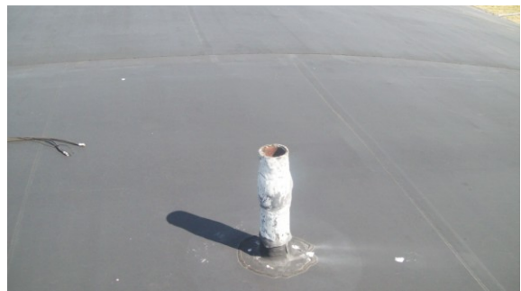
Photo #18: Roof Penetration Tar Sample 30A 3% Chrysotile Asbestos
