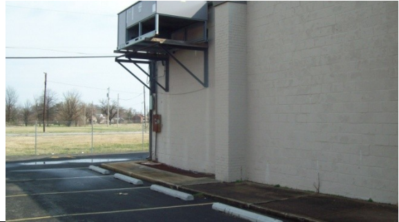
Photo #2: 4646 Exterior Side B LBP on Wall
