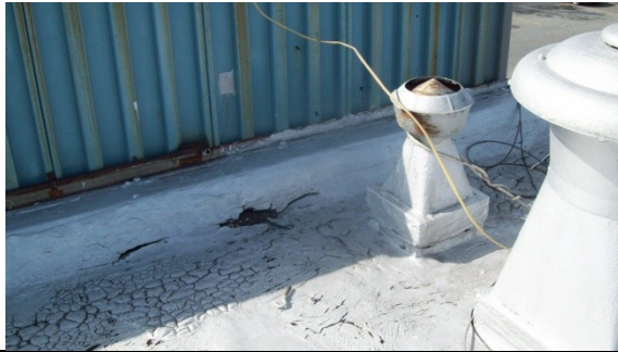
Photo #7: 4670 Roof LBP on Vent Pipes and Parapet Wall
