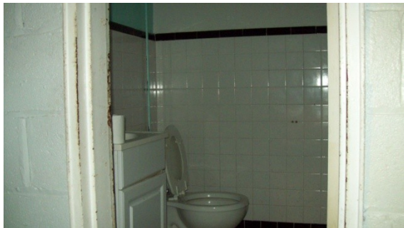
Photo #5: 4646 Basement Bathroom Black Ceramic Border Tile Elevated Lead
