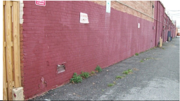
Photo #8: 4670 Exterior Rear LBP on Vent
