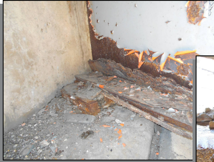
P-0205 - Delamination on beam
