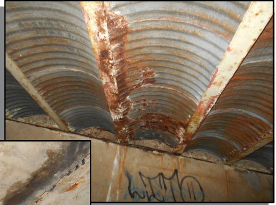
P-0220 - Corrosion on beams
