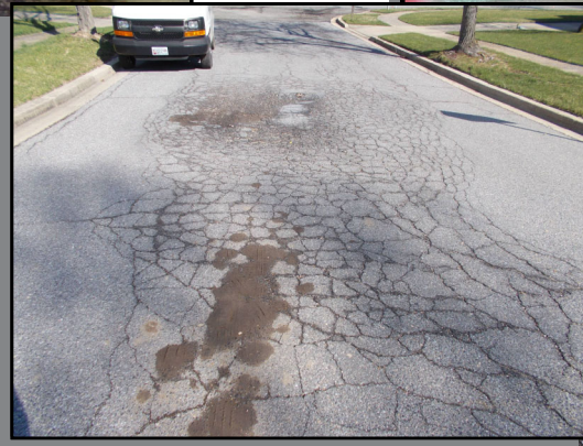
P-0579 - Cracks in the approach pavement
