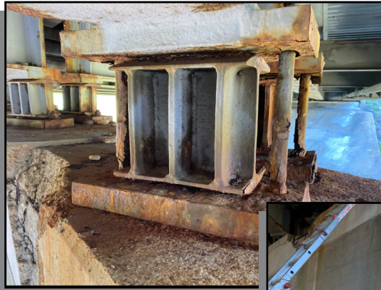
P-0294 - Corrosion on bearing
