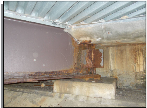
P-0396 - Missing anchor bolt
