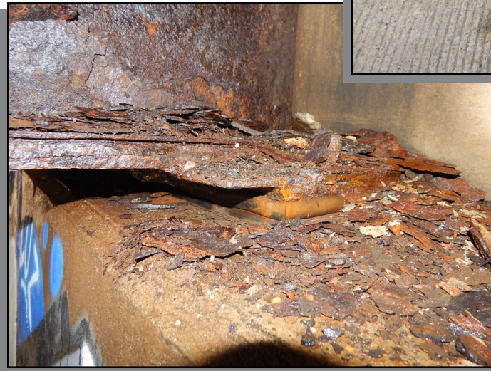
P-0190 - Section loss at beam end
