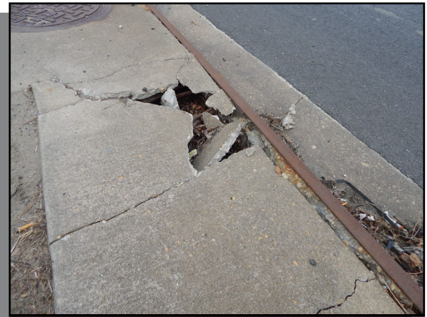
P-0204 - Spall and undermining of sidewalk
