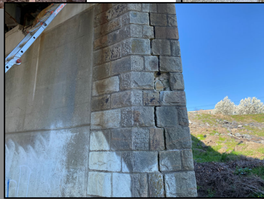
P-0294 - Cracks in masonry of pier nose
