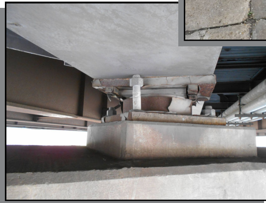
P-0117 - Loose anchor bolt
