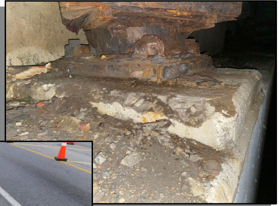
P-0117 - Corrosion on beams
