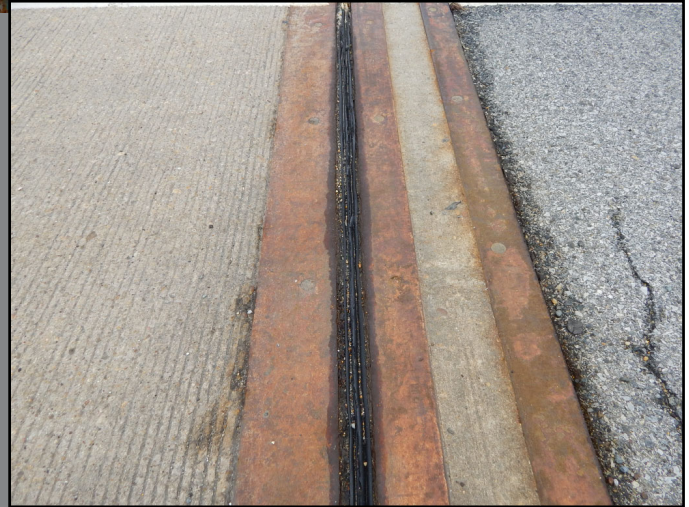
P-0190 - Cracks in compression seal
