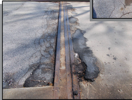
P-0579 - Potholes at the bridge transition
