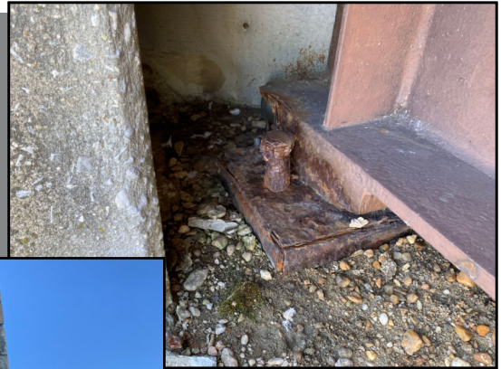
P-0294 - Corrosion on bearing
