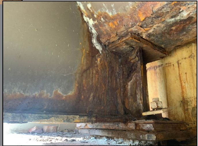
P-0283 - Corrosion at end of beam
