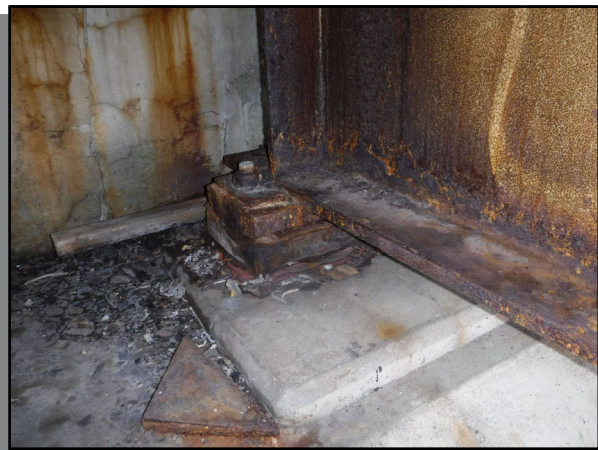
P-0273 - Corrosion on bearing
