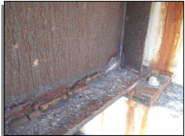
P-0484 - Delamination at beam end
