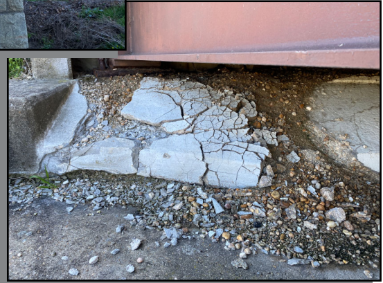
P-0294 - Spalls and cracks in abutment
