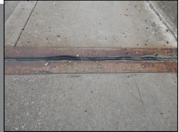
P-0204 - Bulging compression seal
