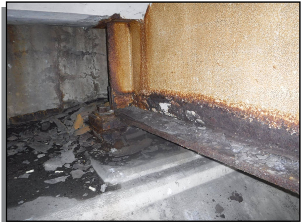
P-0273 - Delamination at bearing
