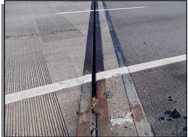
P-0169 - Missing compression seal
