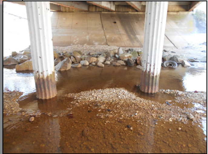
P-0205 - Missing paint and corrosion on piles
