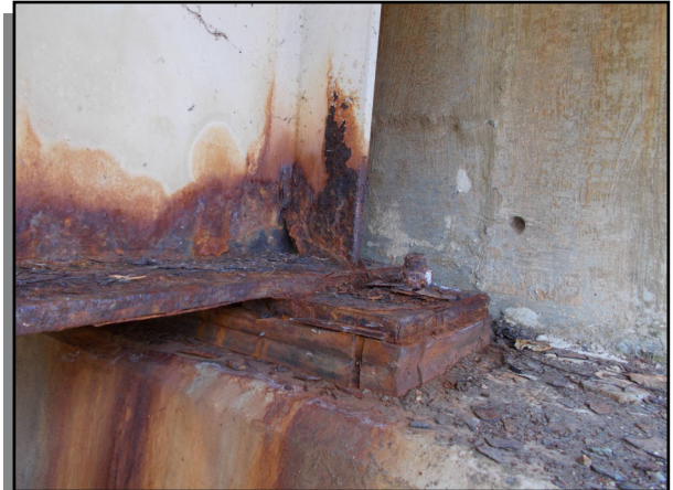
P-0490 - Delamination on bearing
