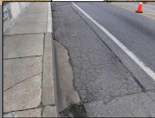
P-0117 - Cracks in approach pavement
