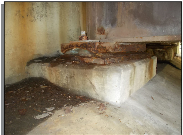
P-0198E - Corrosion on bearing
