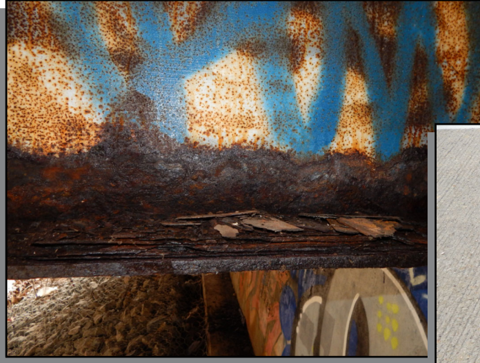
P-0190 - Delamination on beam
