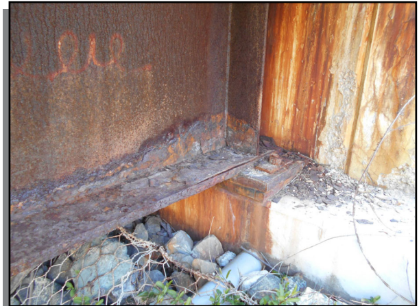
P-0484 - Delamination on bearing
