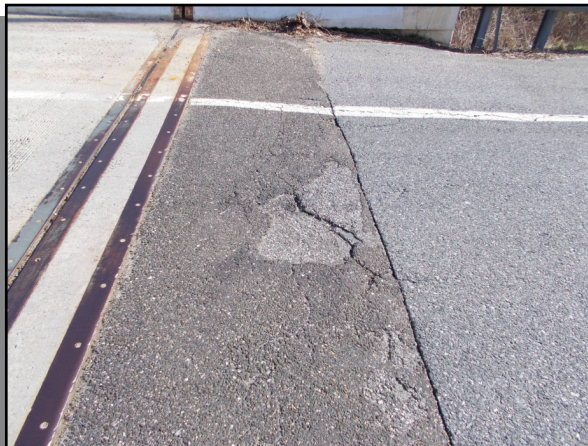
P-0490 - Potholes in the approach pavement
