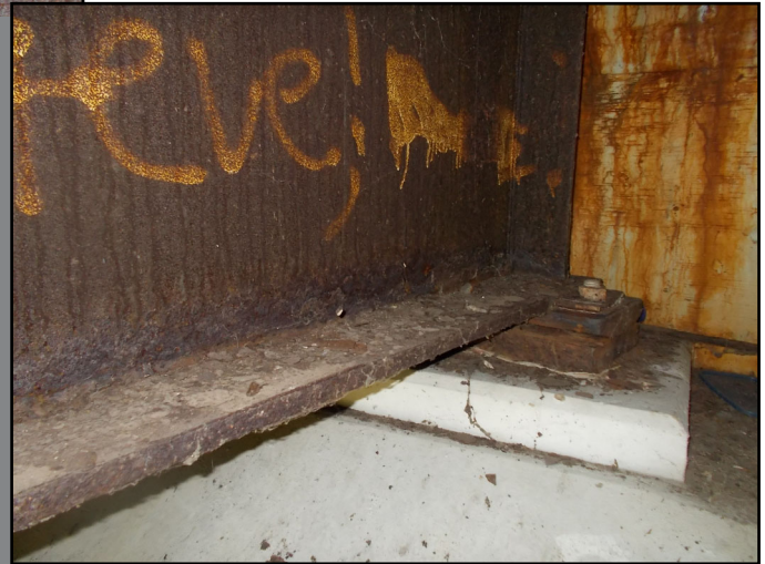
P-0198W - Delamination on bearing
