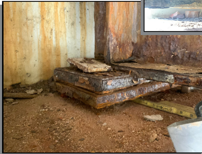
P-0283 - Delamination on bearing
