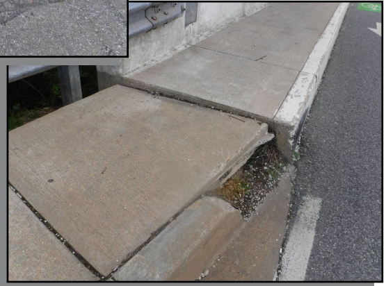
P-0117 - Settlement of sidewalk
