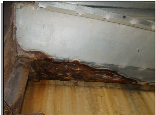
P-0198E - Corrosion below roadway joint
