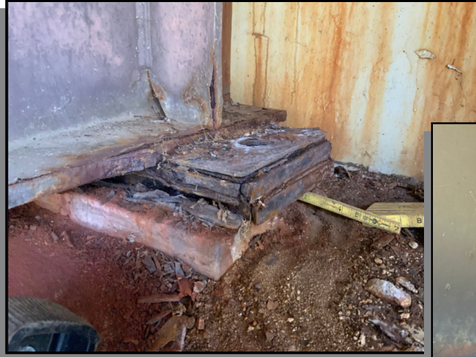
P-0283 - Missing anchor bolt
