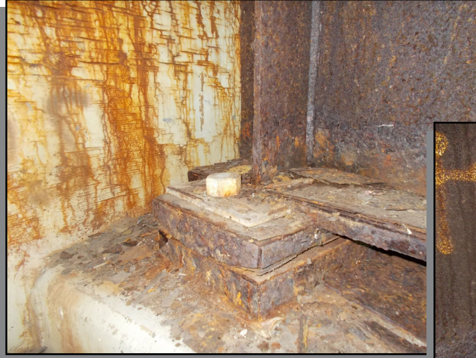
P-0198W - Delamination on beam end
