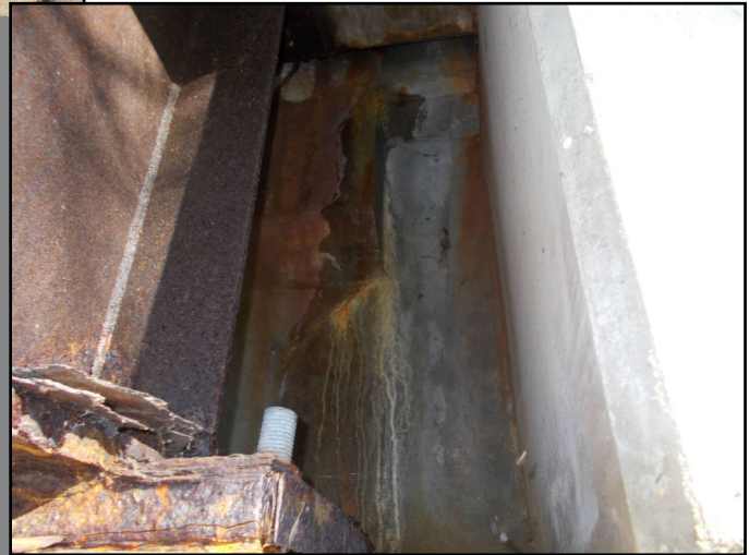
P-0596 - Corrosion at end of beam
