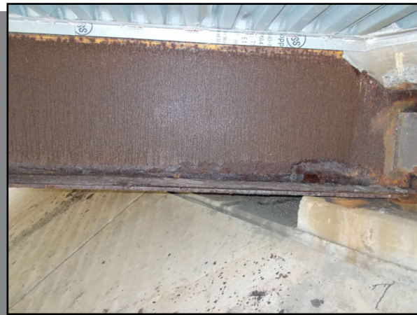
P-0396 - Corrosion on beam
