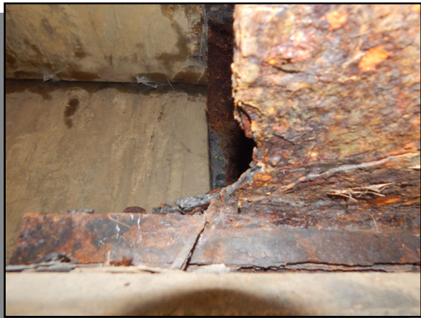
P-0204 - Section loss on beam bottom flange
