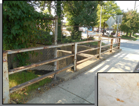
P-0220 - Peeling paint on railing
