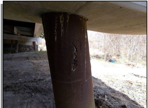
P-0490 - Section loss on pile
