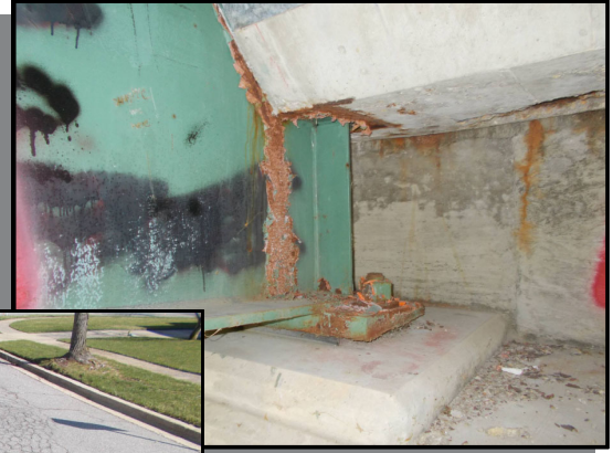
P-0579 - Corrosion on bearing
