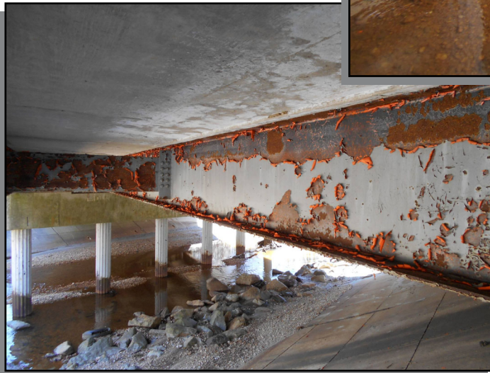
P-0205 - Peeling paint on beams
