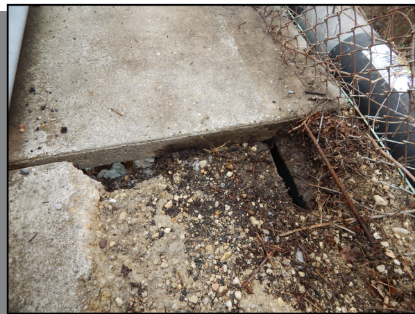
P-0185 - Spall and hole in sidewalk
