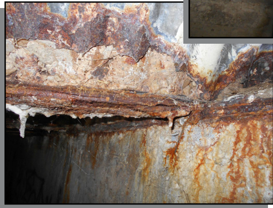
P-0220 - Delamination on beams
