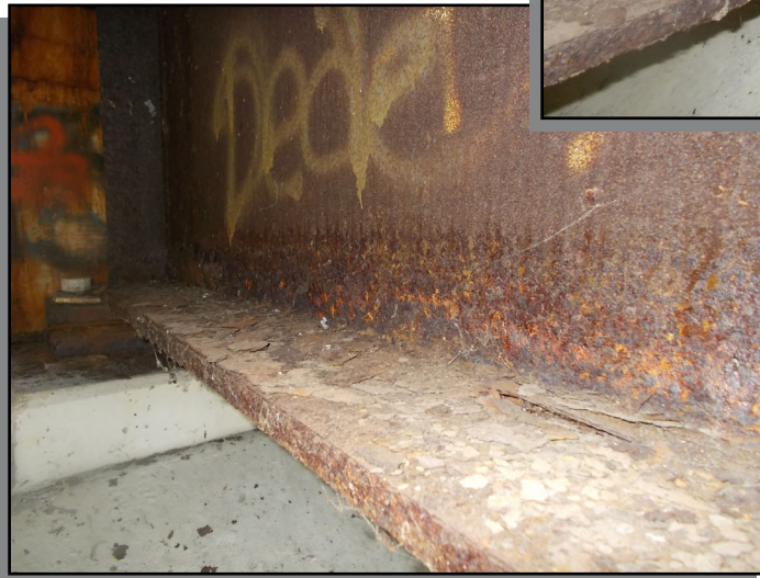
P-0198W - Delamination on beam
