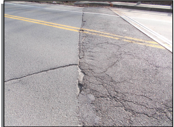
P-0396 - Cracks and potholes in the approach pavement
