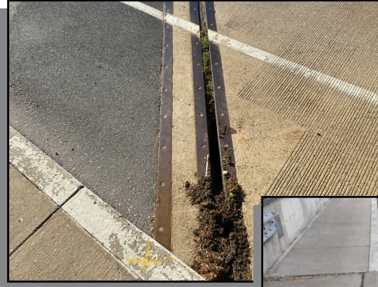
P-0117 - Depressed compression joint
