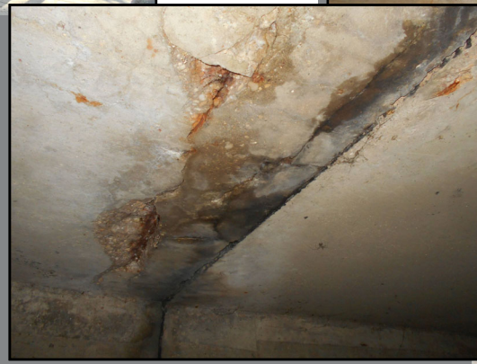
P-0220 - Spalls and cracks in the soffit
