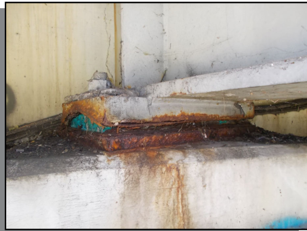
P-0169 - Corrosion on bearing
