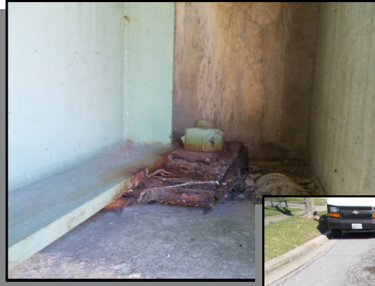
P-0579 - Corrosion on bearing
