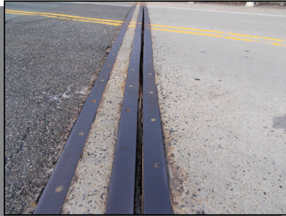
P-0396 - Depressed compression seal
