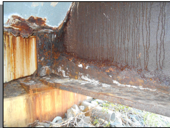
P-0484 - Delamination at beam end
