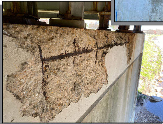
P-0294 - Spall in pier cap
