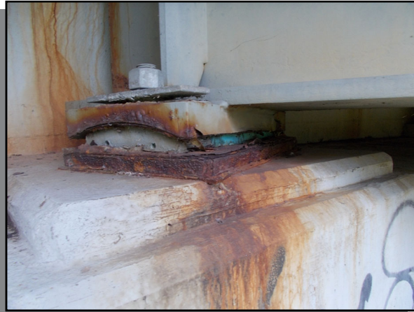
P-0169 - Corrosion on bearing
