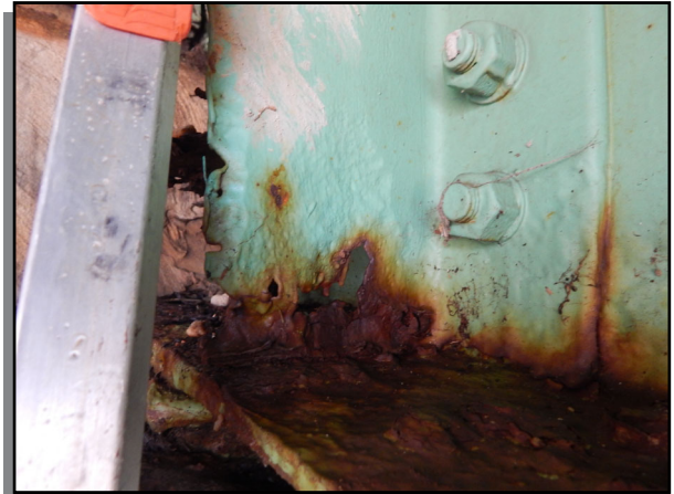
P-0185 - Corrosion at beam end
