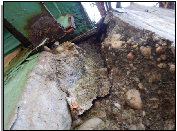
P-0185 - Spall in the abutment
