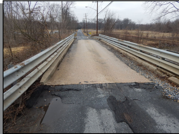
P-0185 - Potholes in the approach pavement
