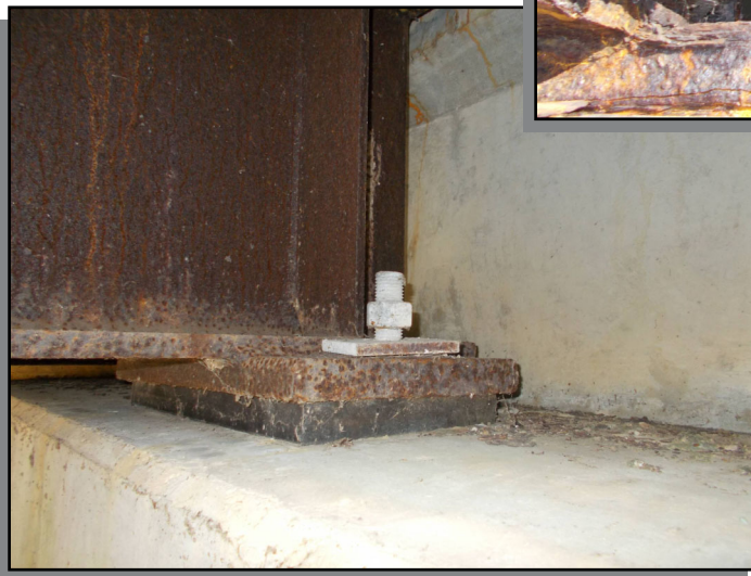
P-0596 - Corrosion on bearing
