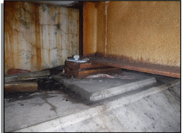
P-0273 - Corrosion on beam end
