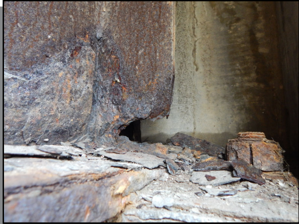
P-0204 - Section loss at beam end
