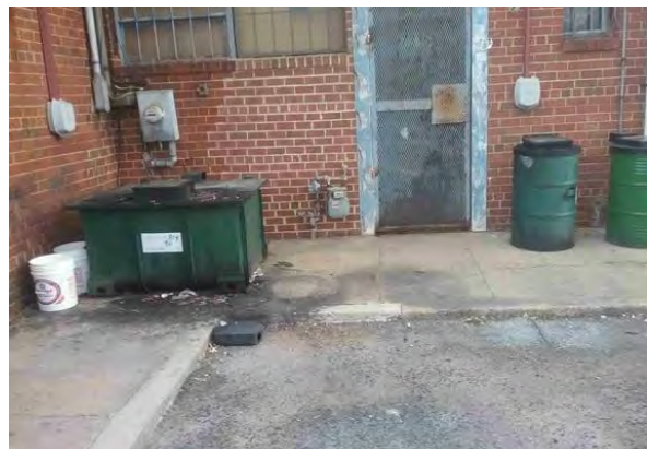
Grease container spillage
